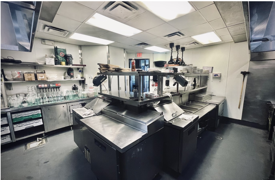
Commercial Kitchen Prep Station
